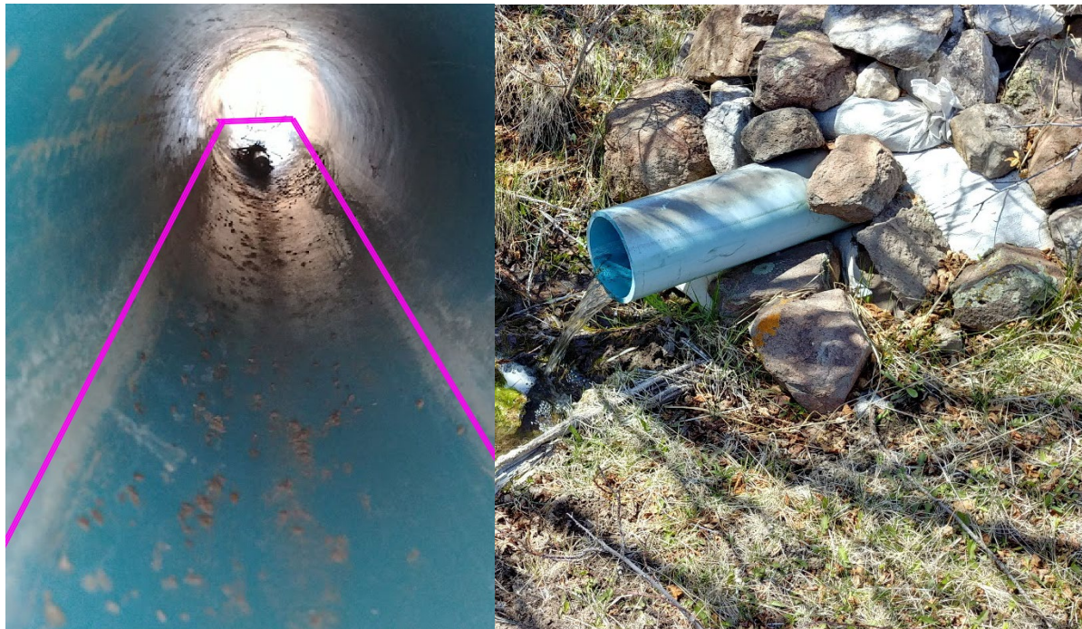
Figure 1.7 This image shows the inside of the flow pipe at the east spill point. Notice the hard water buildup along the walls of the pipe, indicated with pink lines. This would suggest a continuous water level in the pipe of 1.5 inches.
